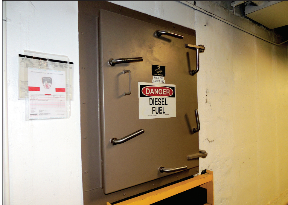
Figure 3-21. Door to a dry floodproofed generator fuel tank vault servicing multiple generators in a high-rise building
