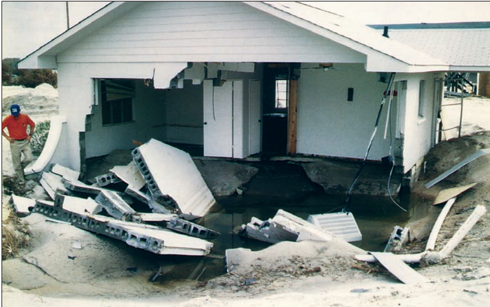
Figure 1-13. Extreme case of localized scour undermining a slab-on-grade house in Topsail Island, North Carolina, after Hurricane Fran (1996). Prior to the storm, the lot was several hundred feet from the shoreline and mapped as an A zone on the FIRM. This case illustrates the need for open foundations in Coastal A zones.
