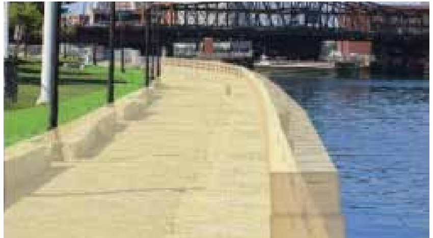
Photos (top and bottom): Climate Resilient Design Standards and Guidelines for Protection of Public Right-of-Way
