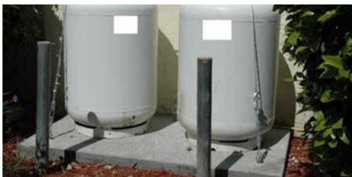
City of Key West, Florida / "Propane Tank Flood Hazards" Photo: Erica Miller
